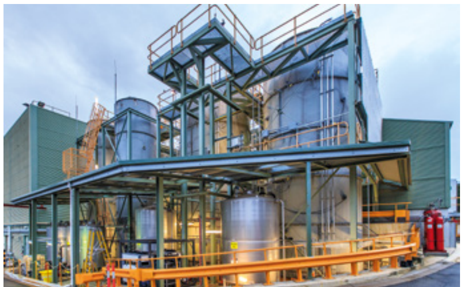
Nuton™ technology pilot plant, Bundoora, Australia.
